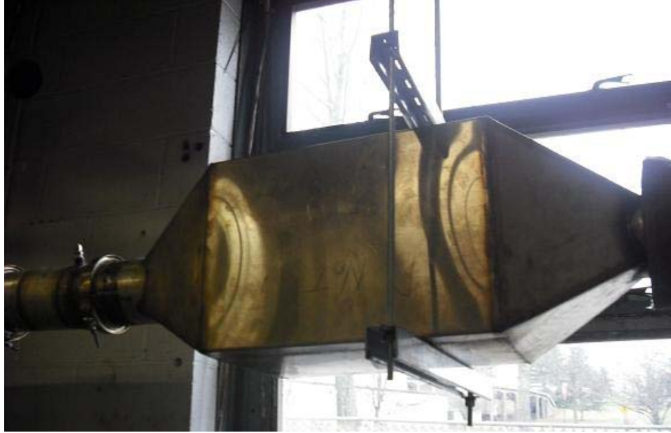
Figure 29. SCR catalyst installed at WVU
