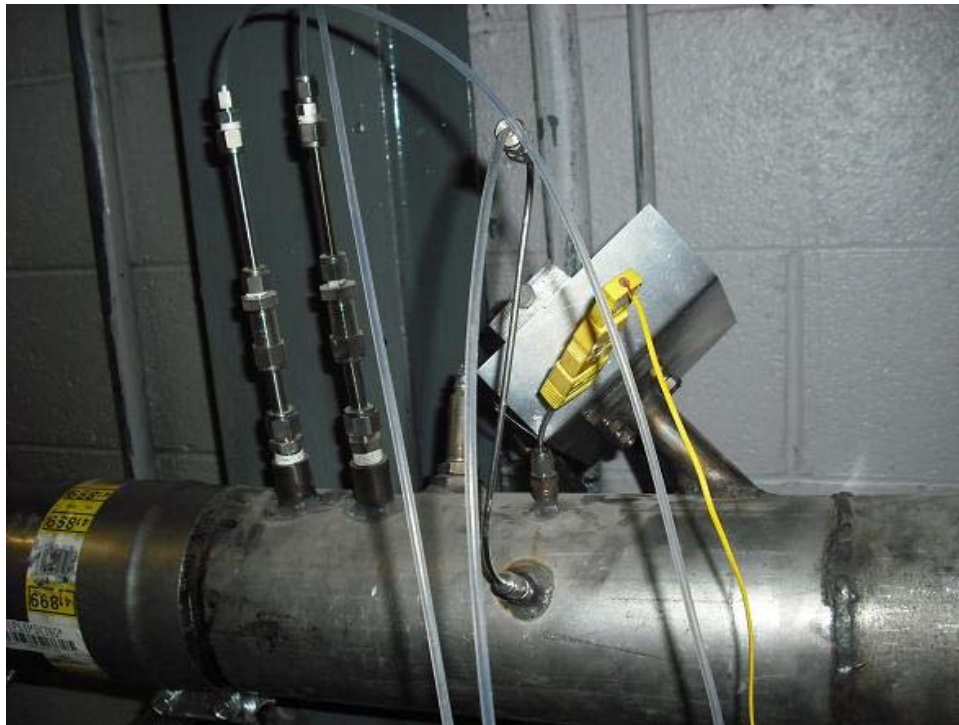
Figure 28. Urea-SCR system installed at WVU
